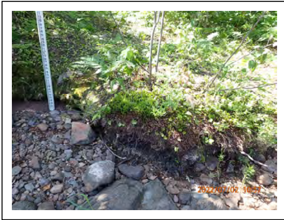
61. Island #13 – Bank erosion
