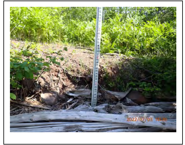
96. Island #20 – Bank erosion
