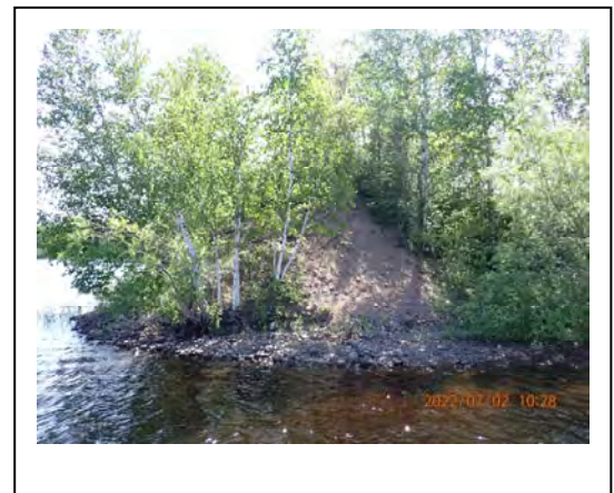
42. Island #9 - Bank erosion
